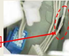
A damaged wire
